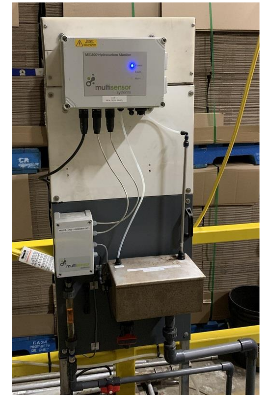
The MS1900 analyzer installed close to the effluent.
